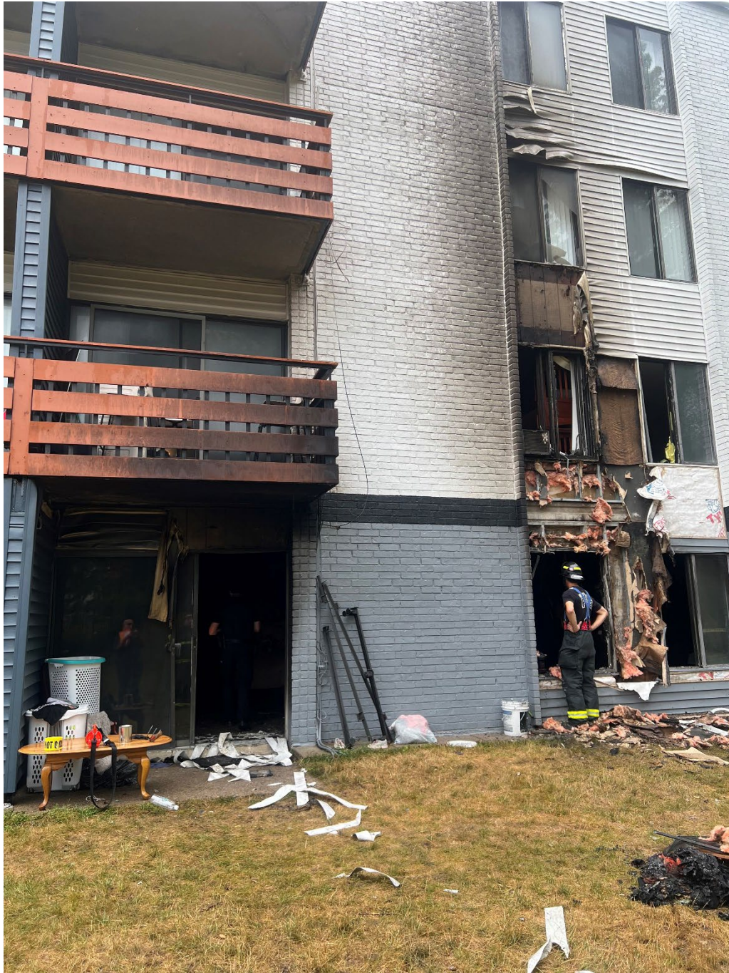
Cutline: A Burnsville firefighter/paramedic assesses damage caused by a fire at the Parkvue Flats Apartments.
